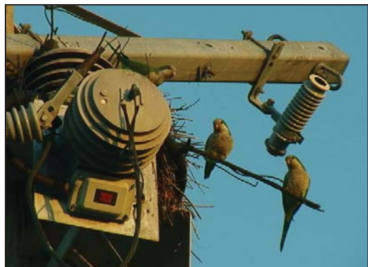
Parakeets nesting in power transformer.
