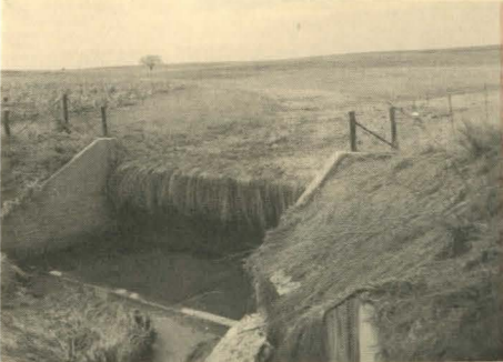
Gullies can be stopped by expensive concrete drops.
